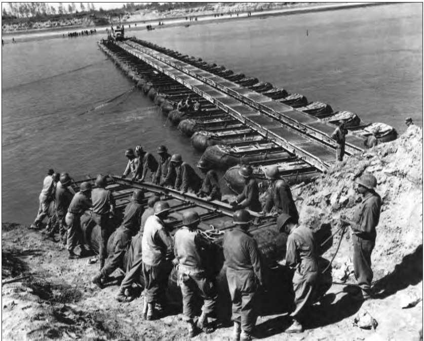
M-2 Treadway Pontoon Bridge under construction across the Po River near Ostiglia (National Archives)
