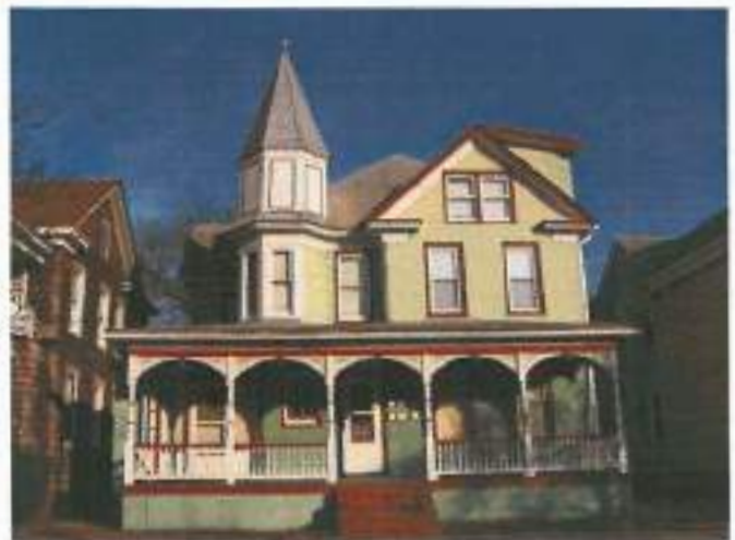
Owners are encouraged to remove modern siding materials like the asbestos shingles on 1333 Chesapeake Avenue and replace them with historically appropriate siding.
