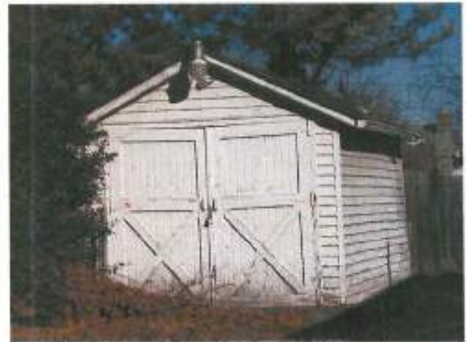
Wooden siding was also commonly used on out-buildings like this garage at 1207 Decatur Street.
