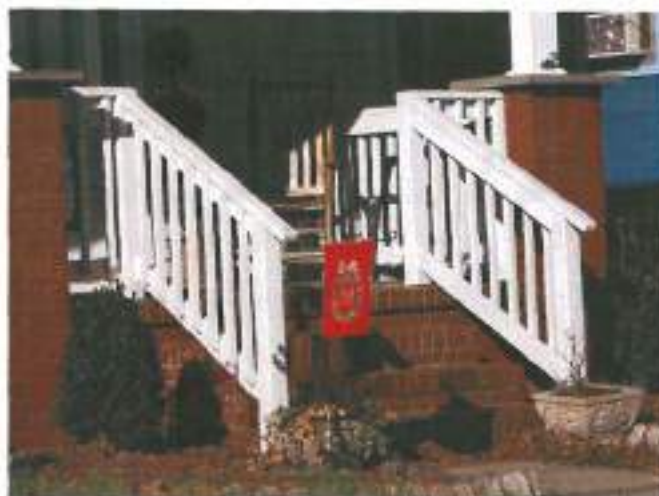
The replacement railings at 1530 Jackson Avenue are appropriate models for most district houses.
