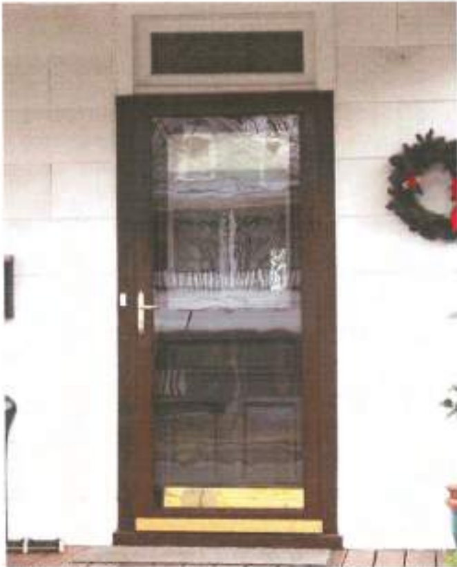
This full-view storm door at 1124 Jackson Avenue is appropriate and enables most of the historic door to be visible, helping retain historic character.
