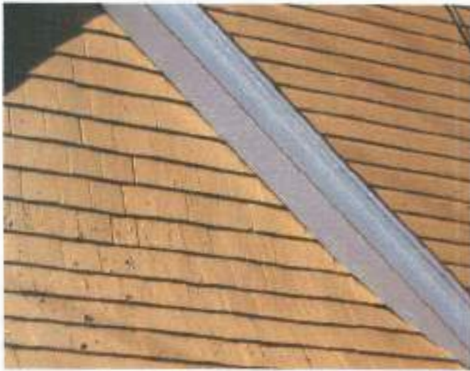
The wooden shingles on 1221 Park Avenue help define the house's historic appearance. If they become damaged they should be repaired in accordance with the guidelines for wood.
